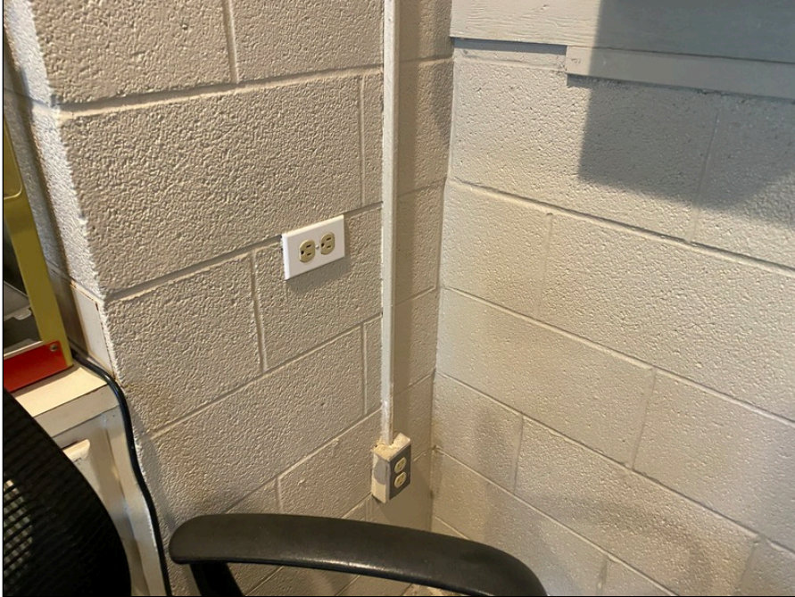
5 - View of lead containing paint in the concession stand.
